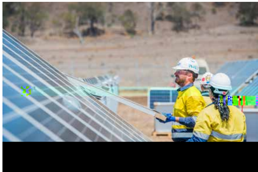
The Warwick Solar Farm will save the University millions of dollars in power costs. Pictured here are workers installing panels on the trackers, which track east to west with intelligent controls to adjust each row individually, rather than all moving as one group. This ensures the best alignment with the sun and better output during all conditions.
